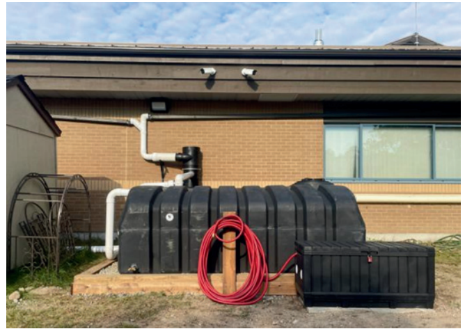
The first rainwater harvesting system was installed at Nbisiing Secondary School in August 2024.
