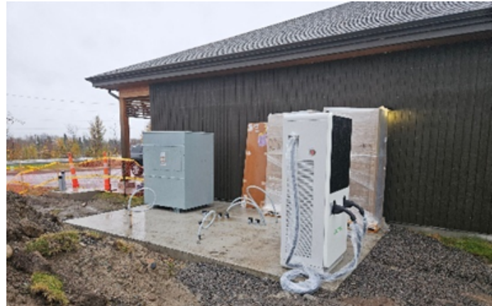
The new Level 3 EV charging station is set to open at Bineshii Business Park in spring 2025.
